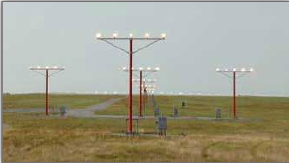
FAA, Lighting System – Medium Approach Light System with Runway Alignment Indicator Lights (MALSR), 2019.
